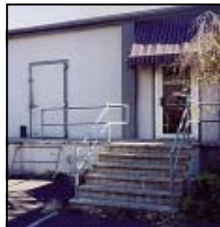
The parking area asphalt and exterior walls of this business are in poor condition. The elements of the asphalt parking area and retaining wall against the sidewalk creates a harsh visual environment. Parking and loading dock areas should be located in an unobtrusive area, if at all possible.
